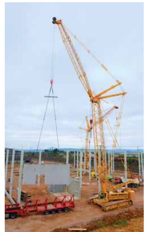
Altogether 1,309 concrete parts with a total weight of 9,700 t will be installed by both crawler cranes.
