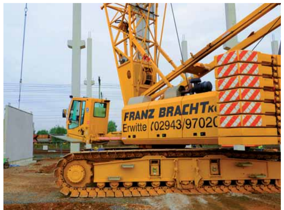
The ability to move under load is also a great advantage at this building site.
