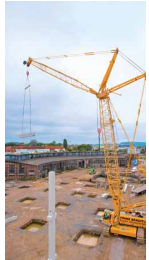
The two SENNEBOGEN 4400 and 5500 crawler cranes installing prefabricated concrete parts for a new furniture retail store. The building in the background is a listed locomotive shed that will be integrated into the furniture store.
