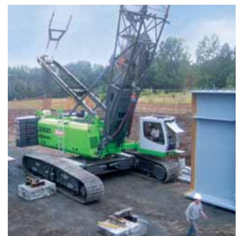
The 3300 crawler crane at Matière is especially for building heavy metal bridges.
