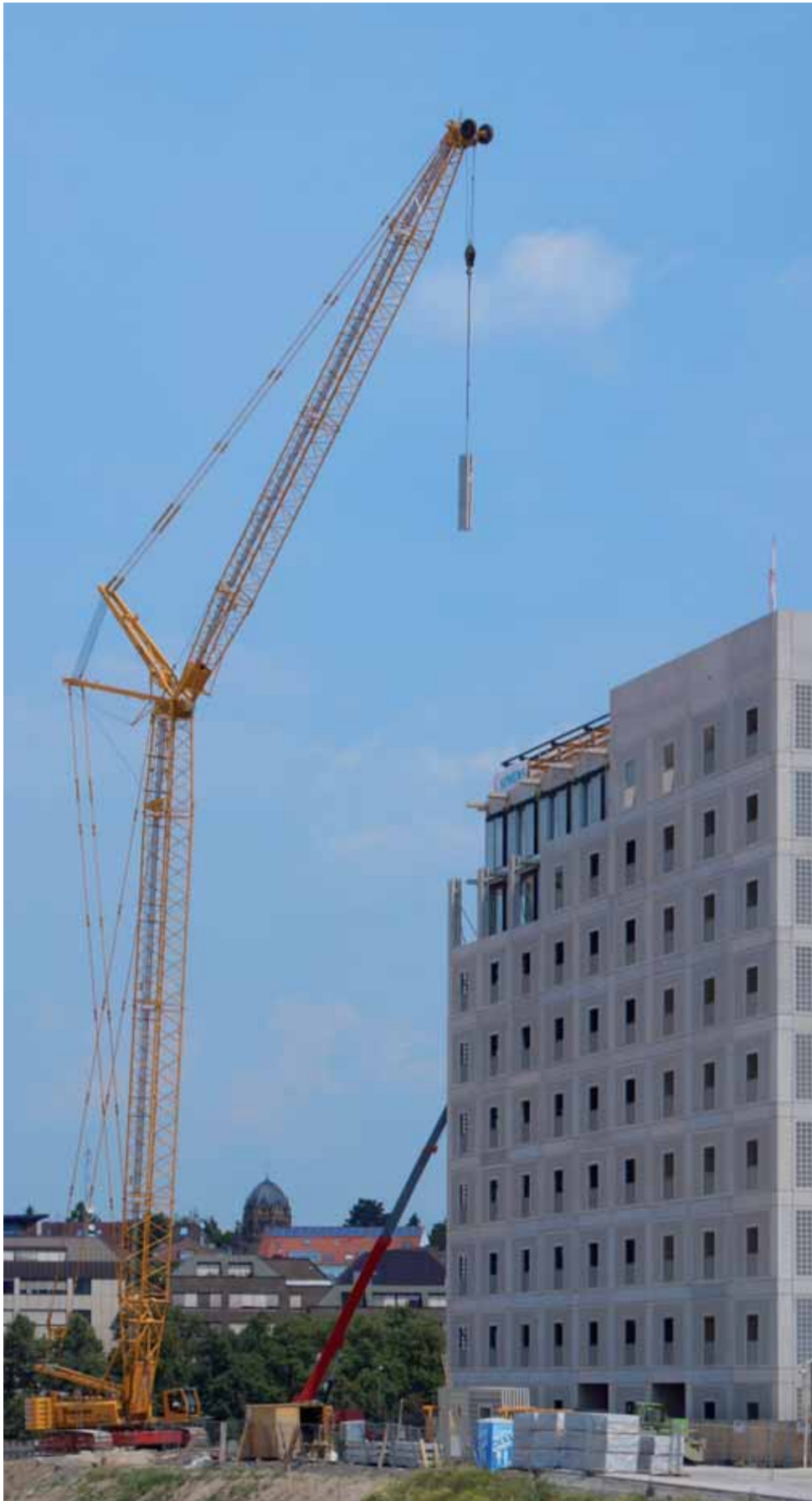
The facade elements, weighing up to 15 t and consisting of concrete and glass building blocks, could be lifted precisely and safely with the SENNEBOGEN 5500 into the desired position.
