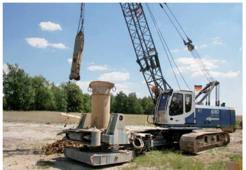
On a 136-km long line section, around 1,000 wells with a depth of 6 to 10 m are being sunk with a new SENNEBOGEN 630 HD.
