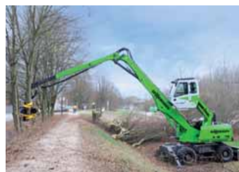
The raised position of the driver is a particular advantage for construction site boundaries and during work over dykes or in ditches.
